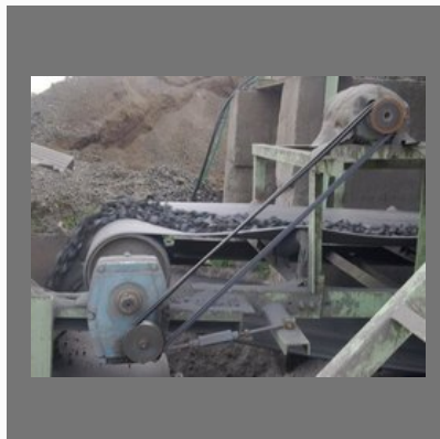
Coal Plant Gearbox
